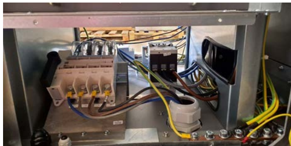
Main disconnect switch for ELECTRA DC STATION 60
