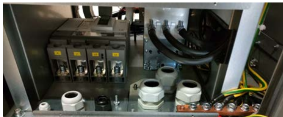
Main circuit breaker for ELECTRA DC STATION 120 and 150
